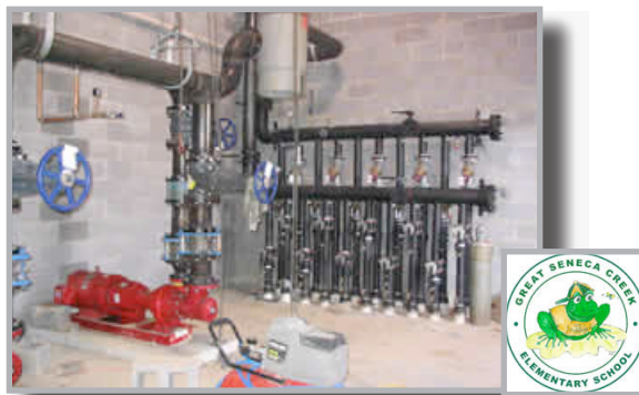
Geothermal Heating and Cooling System Great Seneca Creek Elementary School, Germantown, Maryland
